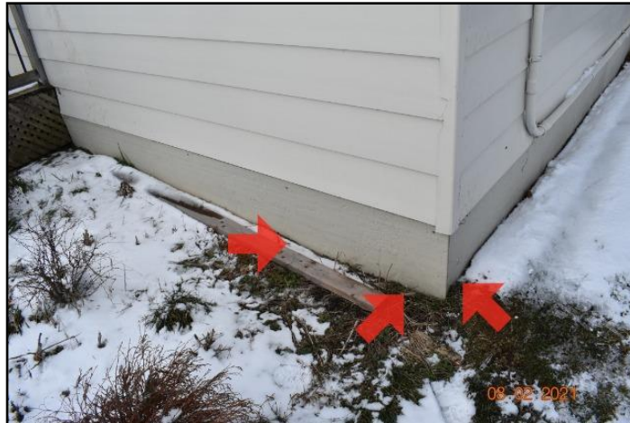
10. Too close to grade
