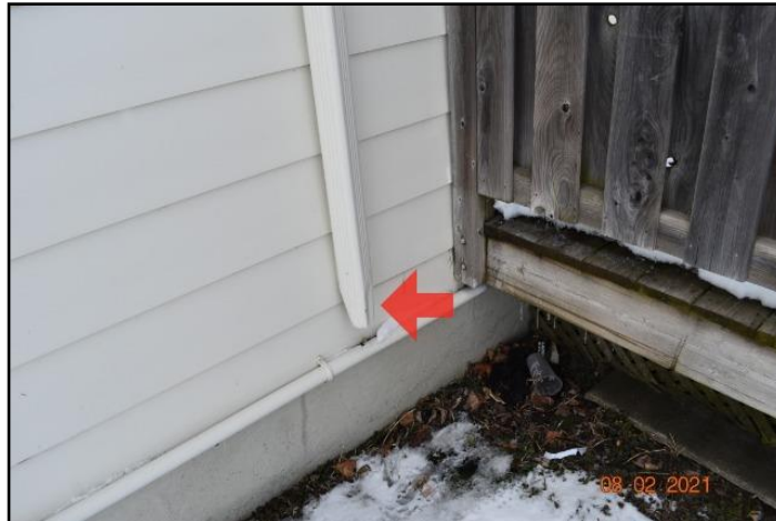
9. Discharge too close to building
