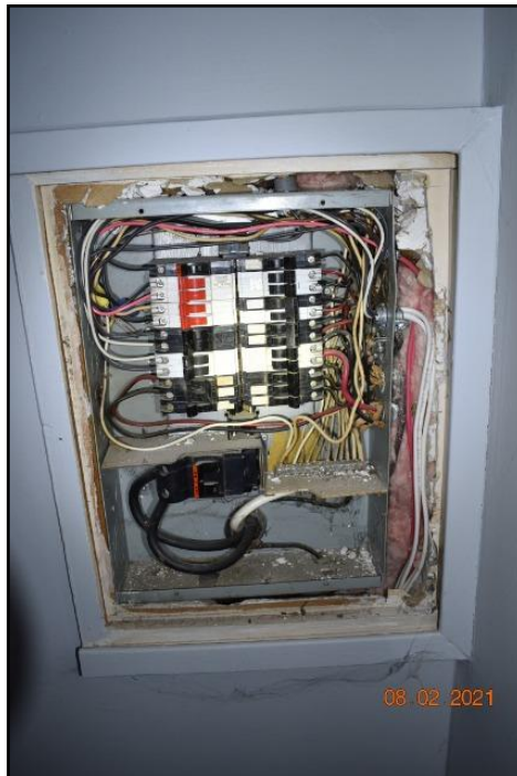
17. Circuits not labeled (Front Unit)
