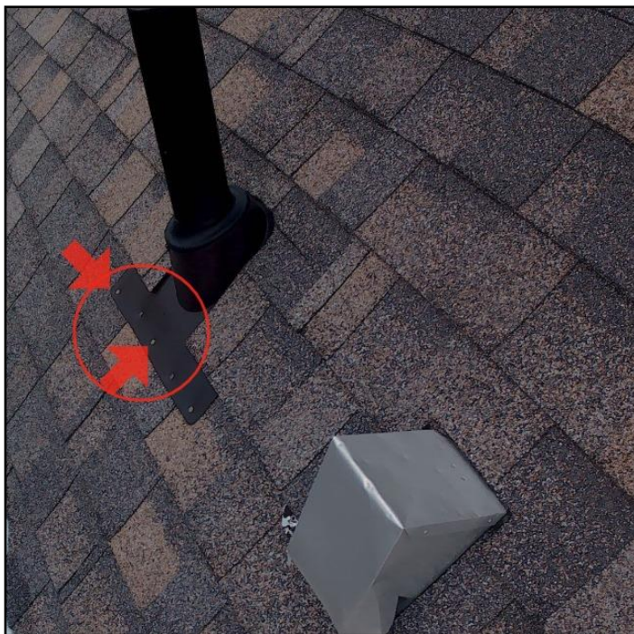
1. Fasteners - exposed / missing
